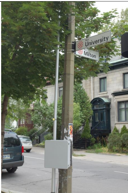
E: Installed Enclosure And Deployed Mast As Seen To Pedestrians. Power System Is Inside Enclosure
